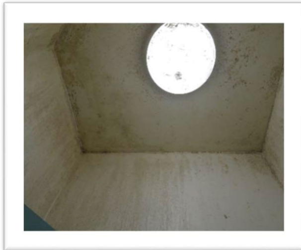
Description: Mould in a cell toilet/shower area
